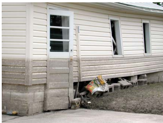
Water lines on the outside of a building are a good indication of the conditions that will be found inside.
